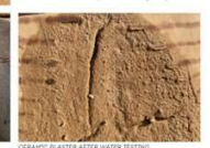
CERAMIC PLASTER AFTER WATER TESTING
